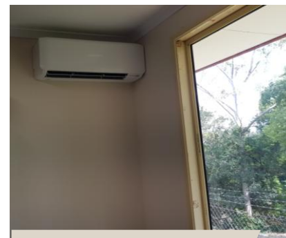
New Office A/C
